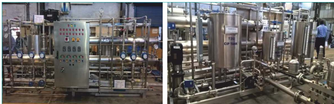
Fig. Pilot plant facility for Micro, Ultra, and Nano filtration modules
