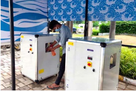
Atmospheric Water Generation at WTP, GIFT City
