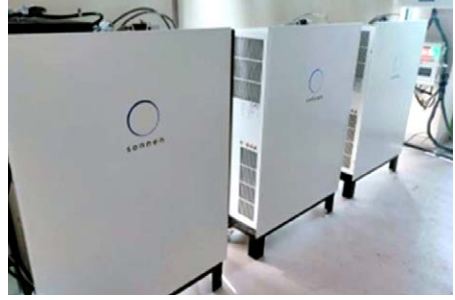
Installed Sonnen batteries at STP, GIFT City
