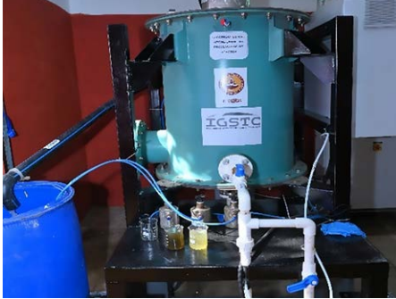
Electrochemical Ozone Oxidation Process (ECOOP) installed at CETP, Tiruppur
