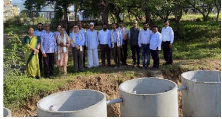
TRC STP installed at Samatha Vidyalaya, Pune
